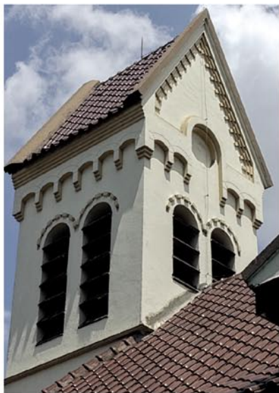
This tower functioning as an air circulation.
